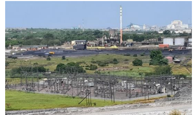
High voltage switchyard
