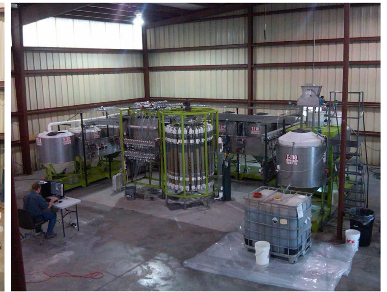
Pilot Plant System for Hydrometallurgical Application
