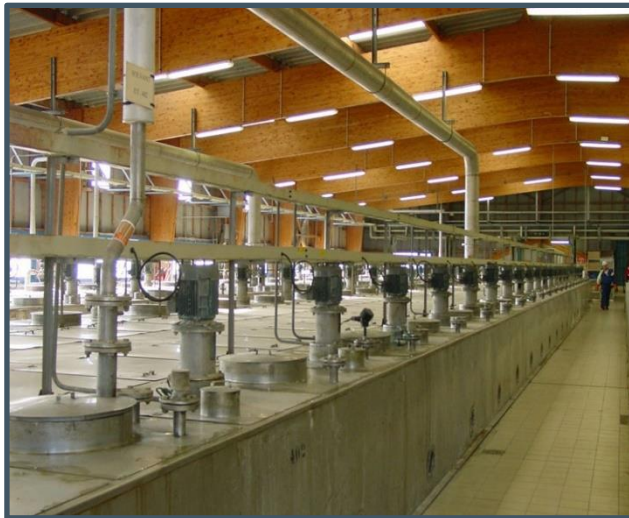
Rare Earth SX separation battery in La Rochelle, France; just one small fraction of overall process
