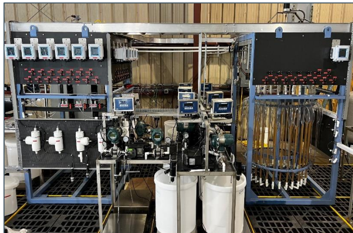
CIX / CIC units at the back-end pilot plant
