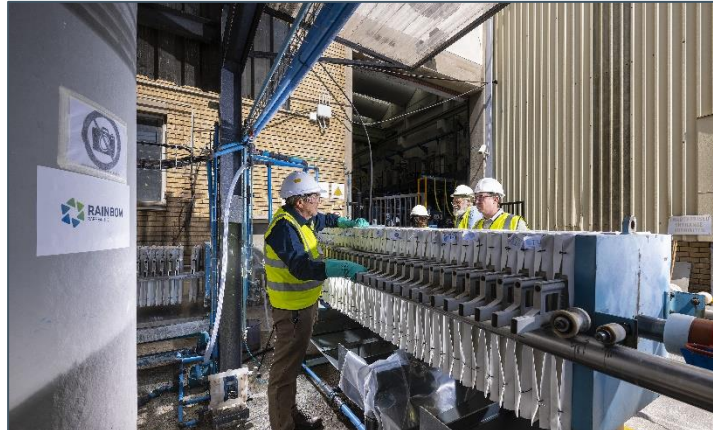
Filter press at the front-end pilot plant
